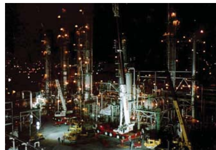
6. Acid gas removal area. A night shot of activity in the acid gas-removal area of Kingsport during the last triennial maintenance/inspection blitz. Courtesy: Eastman Chemical Co.
