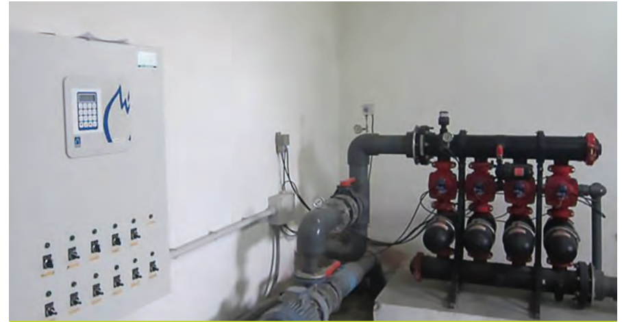
Central control unit to program irrigation time and flow
